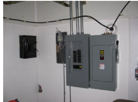
Radio Tower / Projection Room Power Panel
