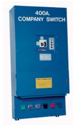
Typical Company Switch
