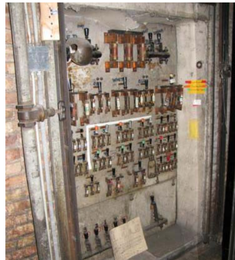
Stage Right Theatre Switchboard
