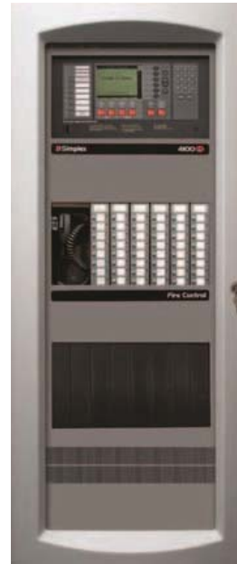
Fire Alarm Control Panel
