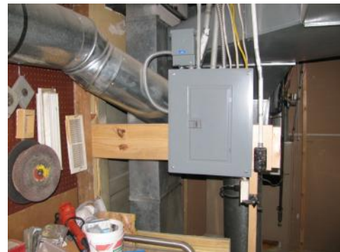
West Mechanical Room Load Center
