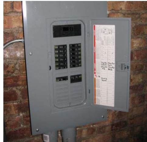
Stage Left Auxiliary Power Panel
