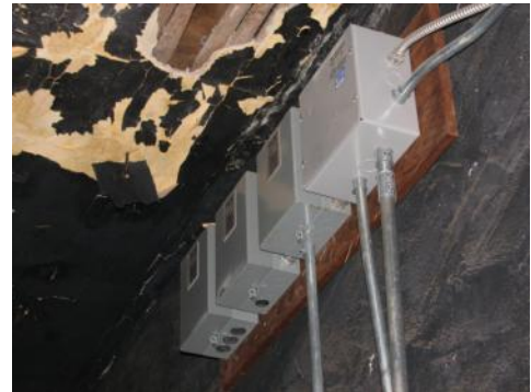
Marquee Lighting Contactors
