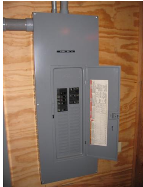
Basement Air Conditioning Power Panel
