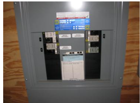
Basement Main Distribution Panel
