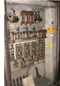
Existing lighting control panel
