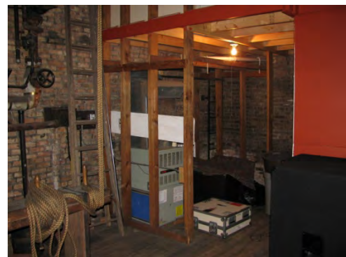
Existing furnace installed on stage=right
