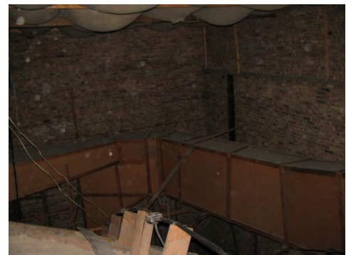
Existing supply air ductwork in Auditorium (House-right)
