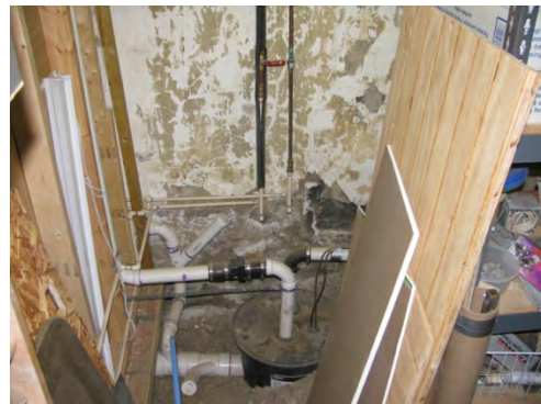
Existing sump pump/sewage ejector
