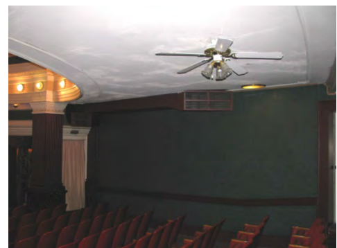
Existing supply air ductwork in Auditorium (House-right)
