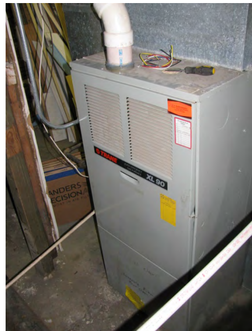
Existing basement furnace
