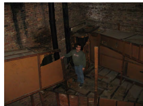
Existing supply ductwork above Auditorium
