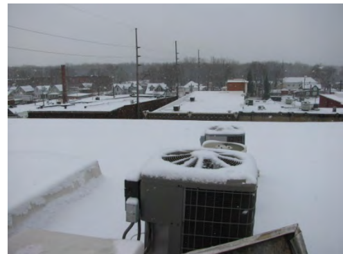
Existing air-cooled condensing units on roof
