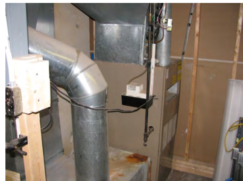
Existing basement furnace
