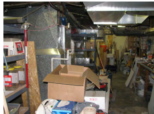
Existing workshop (multiple furnaces installed)
