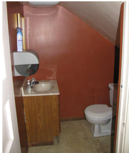
Existing typical plumbing fixtures
