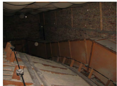
Existing supply ductwork above Auditorium
