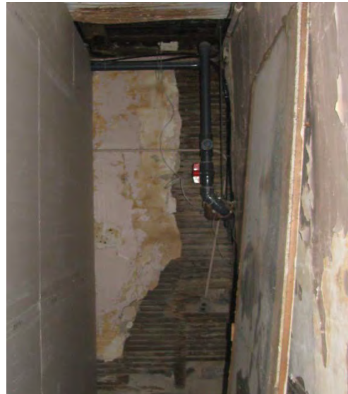
Existing domestic water service
