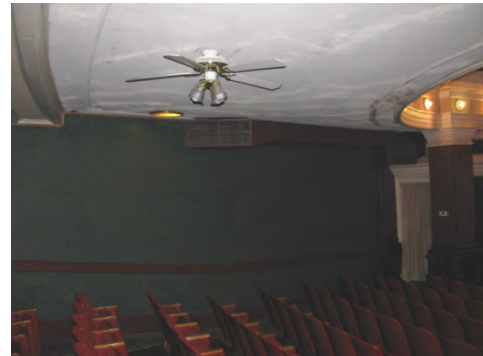
Existing supply air ductwork in Auditorium (House-left)
