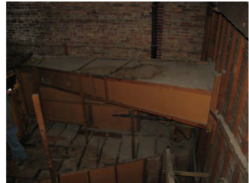
Existing supply ductwork above Auditorium
