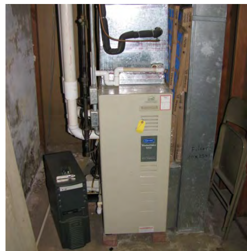
Existing basement furnace
