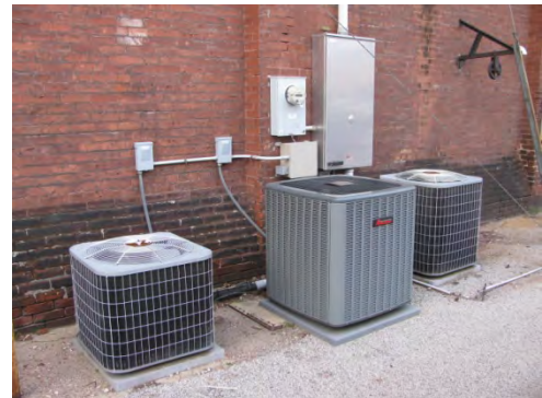
Existing air-cooled condensing units in alley
