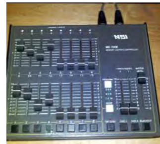
Existing front wash lighting controller
