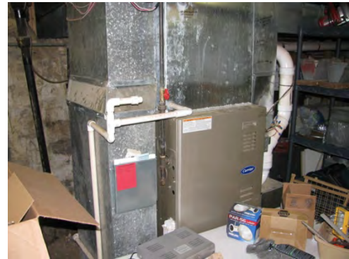
Existing basement furnace
